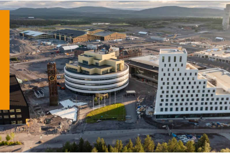
FIGURE A1.38 The new town centre buildings under construction in the new part of the town in the east.
